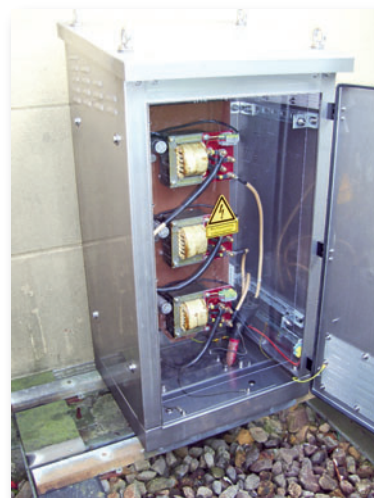
Audio-frequency lock 3-phase 6 kV, 495 Hz
